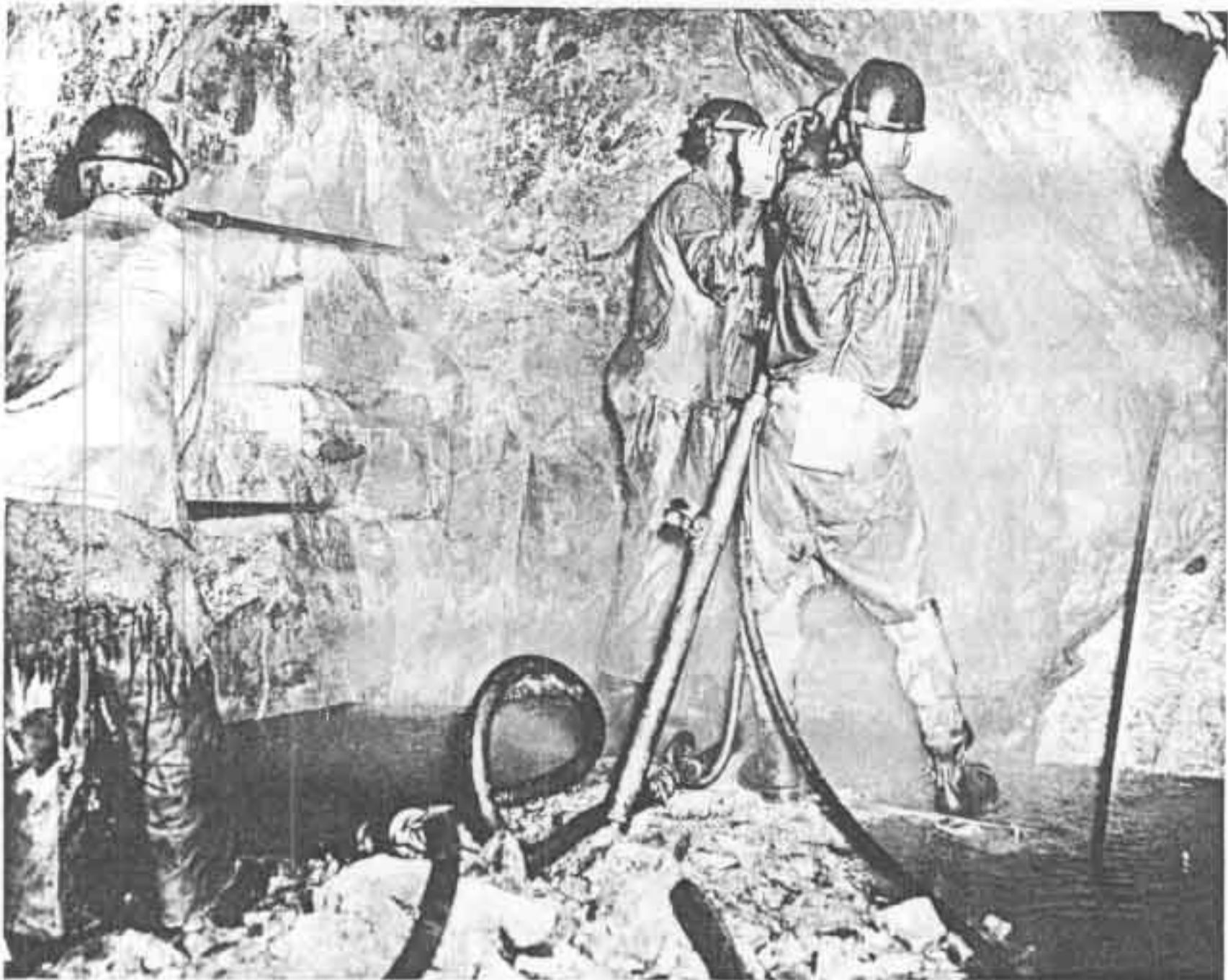
Figure 128. The copper belt of Northern Rhodesia is one of the world's chief sources of copper, the largest in the Commonwealth and the third in the world. There are four producing mines at present and more are being developed. Shown here is the Roan Antelope Copper Mine in Northern Rhodesia. (Courtesy of Federal Information Department, Southern Rhodesia.)
