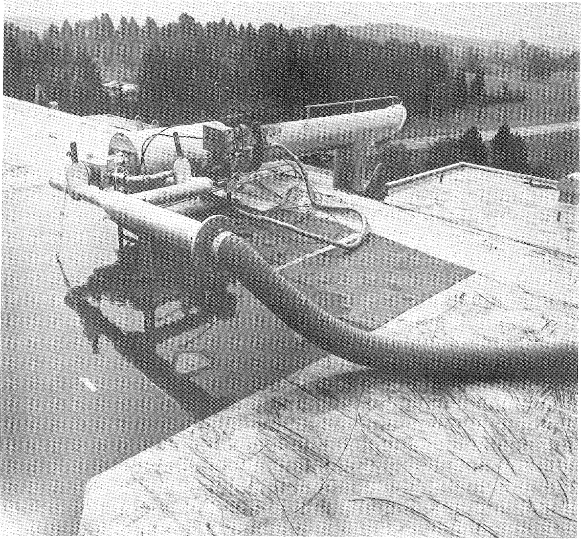
Figure 5. Detail view of gas burner in spray concentrator for fish stickwater.
