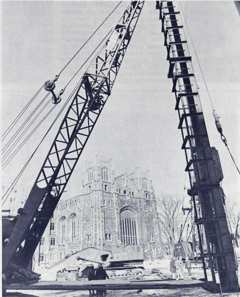
GETTING DOWN TO BUSINESS —The construction area of the below-grade Law Library addition will eventually become a landscaped park.
