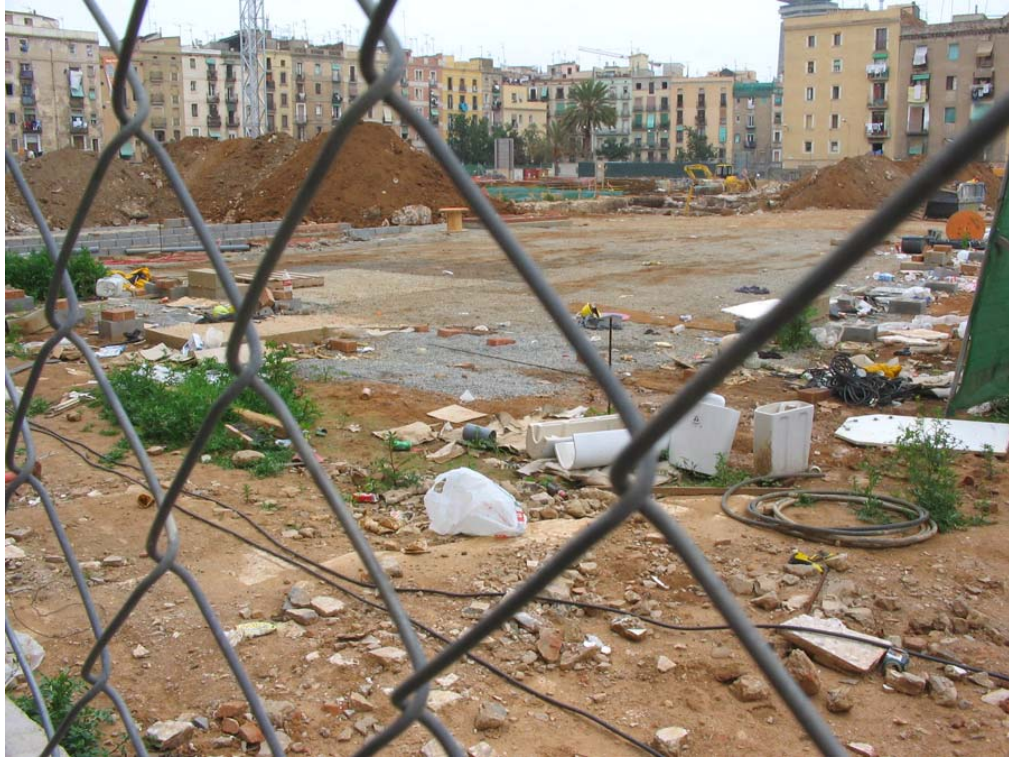
Fig. 1.22. Seized gap in the Raval where a five star hotel is being built. Megan Saltzman, February 2005.
