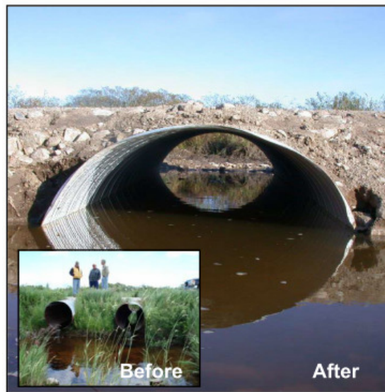
Figure 6.5. Before and after shots of a culvert crossing improvement project on a St. Marys River tributary. The project greatly improved fish passage from the tributary to the river/marsh complex. (Before photo by Neal Godby, after photo by Andrea Ania).
