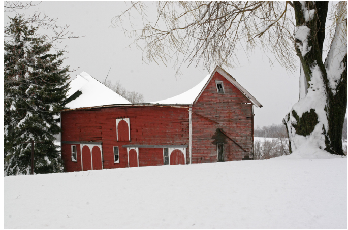
Figure 7. Collapsing barn in Lodi Township, Michigan
