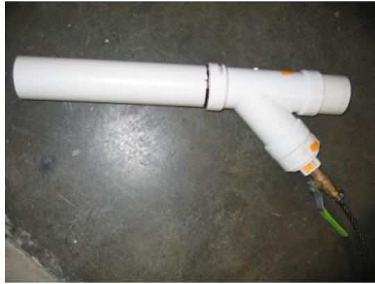
Figure 87: Water Injector Tee Connection
