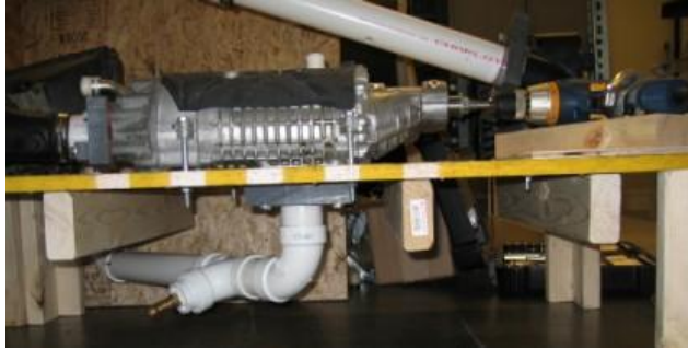
Figure 84: PVC Ductwork After Compressor Outlet
