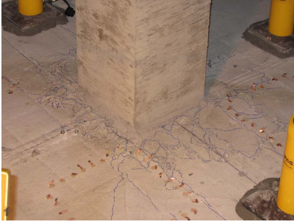
Fig. 4-16 Connection Damage in Specimen SU2 after Test (5/8 Gravity Shear Ratio)
