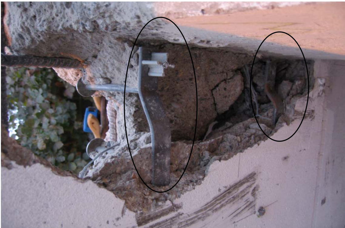
Fig. 5-26 Damage in Shear Stud Reinforcement of Specimen SB3 after Removal of Connection Concrete (Notice "Tunnel" of Concrete Left by Second Shear Stud)
