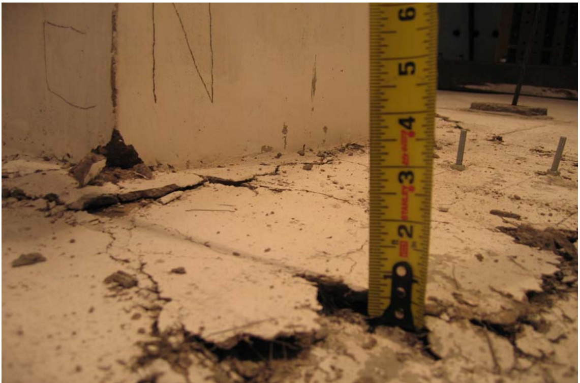
Fig. 5-22 Half-inch Vertical Settlement of Slab in Specimen SB2 after Punching Shear Failure
