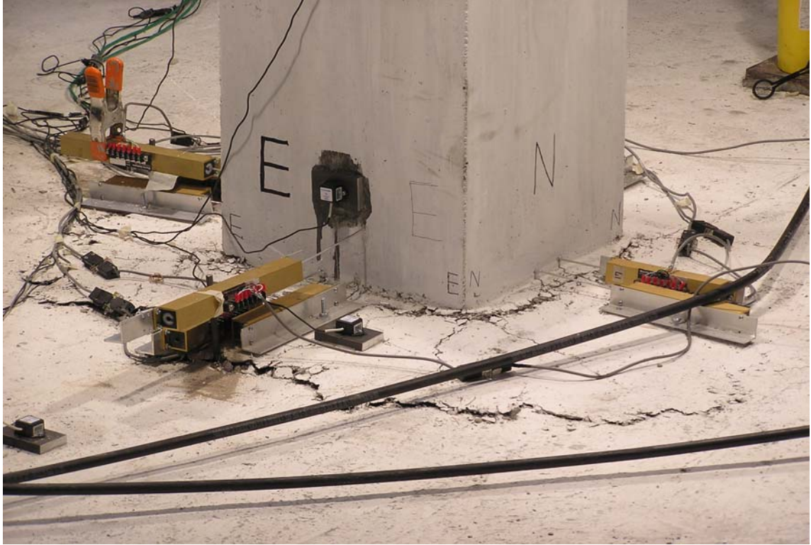
Fig. 5-18 Initiation of Punching Shear Failure in Specimen SB1
