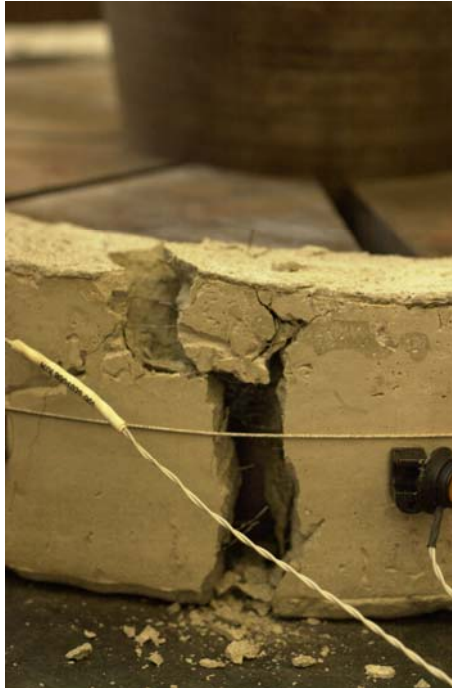
Figure 8.7: Localization crack of Hooked specimen
