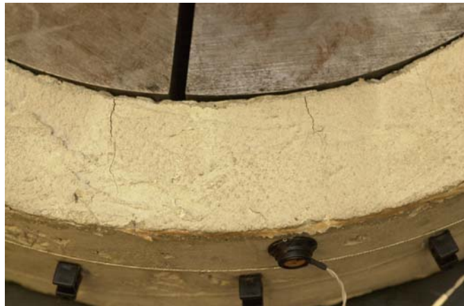
Figure 8.10: Multiple cracking for both inside and outside surface of specimens
