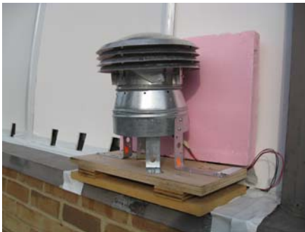
Figure 4.33 Exterior Weather Station
