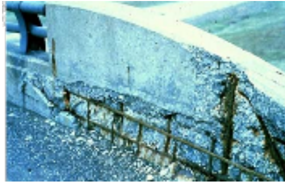
Deterioration due to steel corrosion, concrete cracking and spalling
