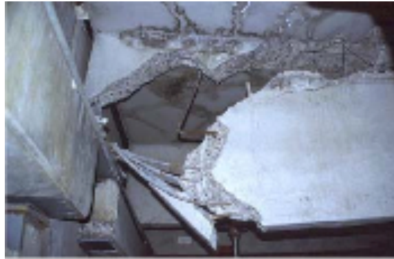
Damage caused by earthquake
