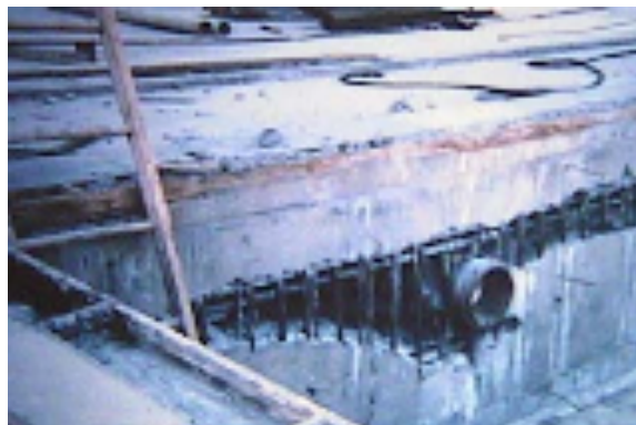
Defect associated with improper detailing and construction practice
