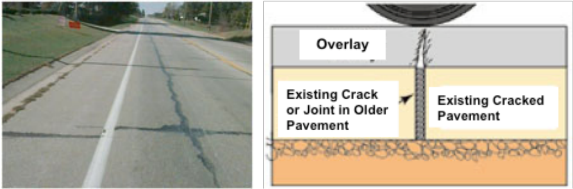
Figure 1.6 – Pavement overlay reflective cracking.
