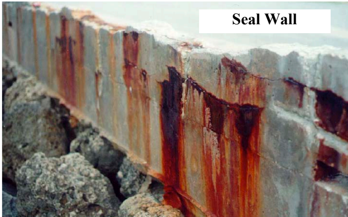
Figure 6.1 – Corrosion in Concrete Structures.
