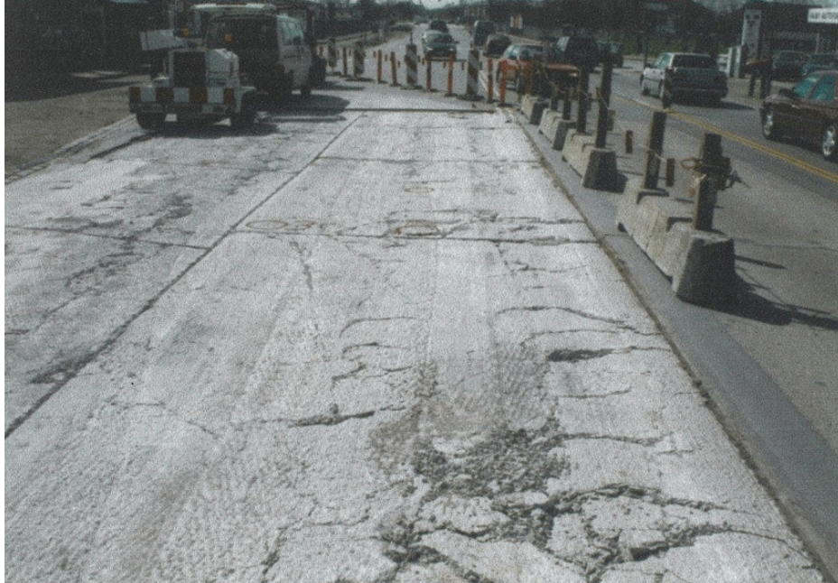
Figure 5.1 – Crack-and-sealed pavement surface.
