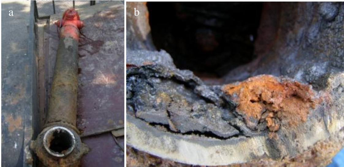
Figure A.1 Drinking water distribution system sampling. (a) Fire hydrant with connection to main line and (b) close-up of main line pipe and biofilm interspersed with pipe corrosion.
