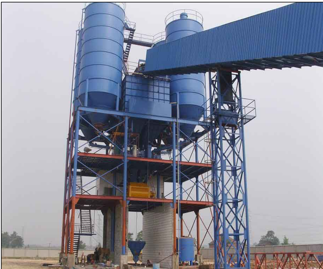
Figure 5-4. Concrete mixing plant bins
