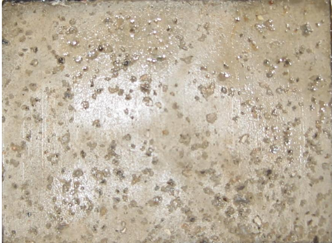
Figure 2- 11 The concrete surface after 5CDF cycles in 3% NaCl solution
