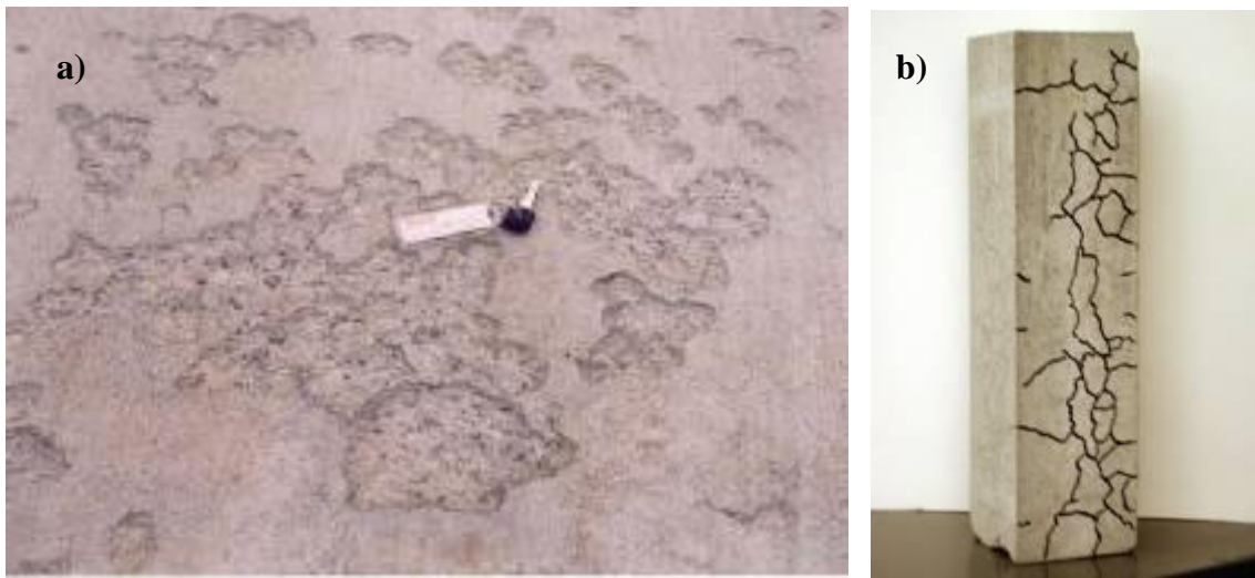
Figure 1- 1 a) Example of salt-scaling damage, b) Example of freeze-thaw damage
