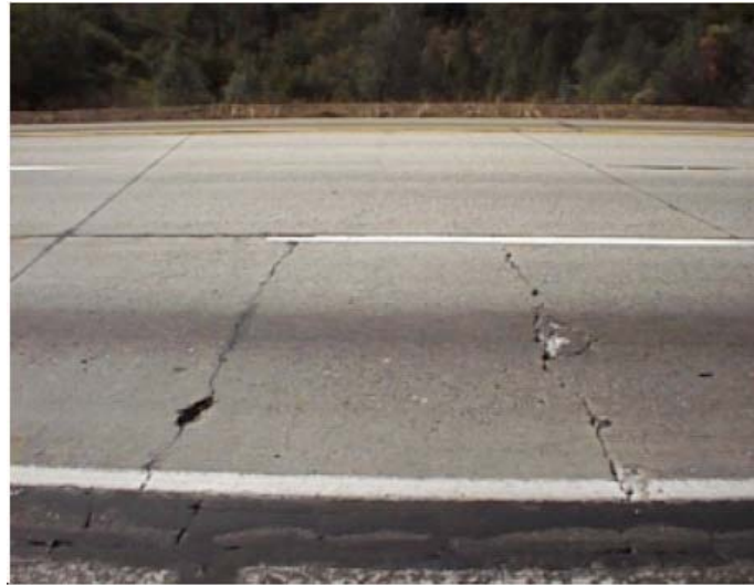
Figure 1: Fractured concrete pavement slab due to repeated loading [3]
