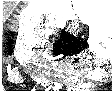
Figure 1: Fracture failure of concrete near steel bolt near column base of a structure during the Kobe earthquake [2]
