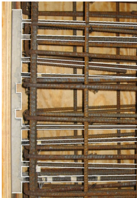
Figure 3.4 – Precast coupling beam embedment. Coupling beam reinforcement (highlighted) is developed parallel to the transverse reinforcement in the wall
