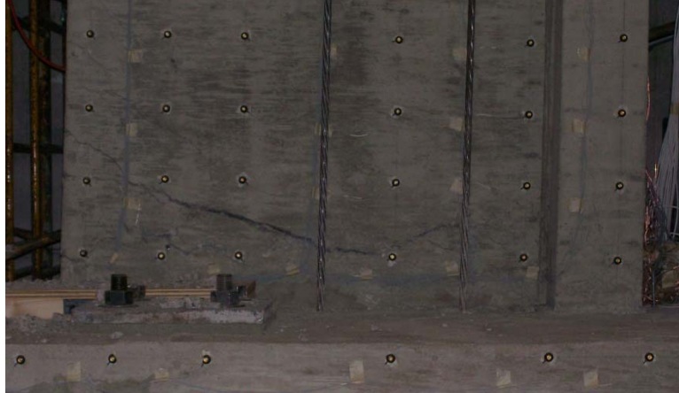
Figure 5.8 – Photo of the base of the wall showing flexural cracking that localized at the termination of the dowel bars extending from the foundation
