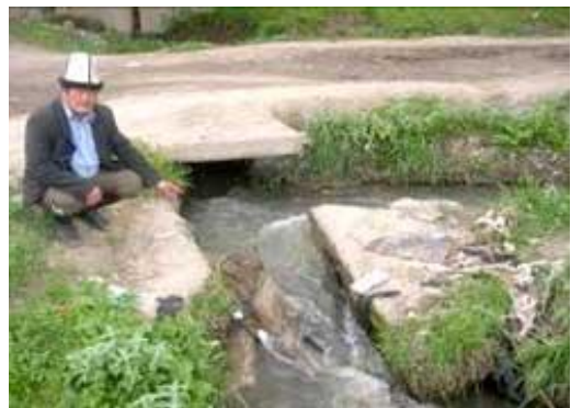
Figure 2.2. Deteriorated canal (WUASP 2010)
