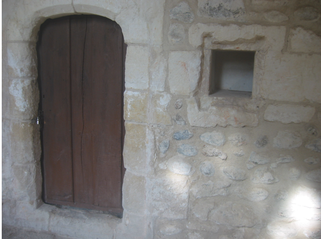
Figure 3.21. Charterhouse of El Paular, monks' cloister, door to former cell and guichet .
