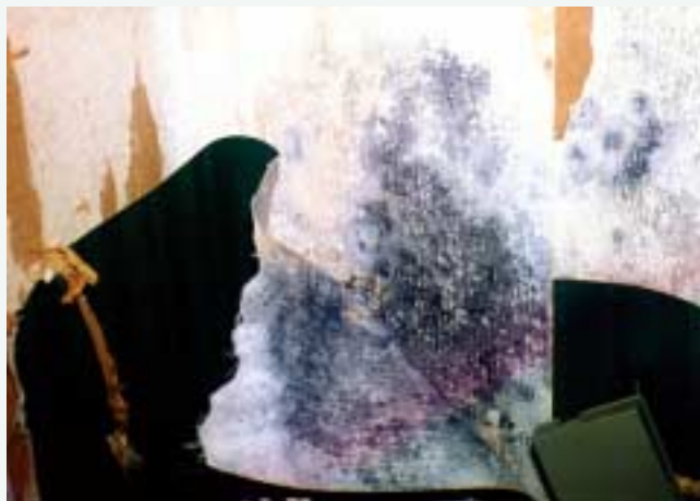
Mold growth behind wallpaper.
