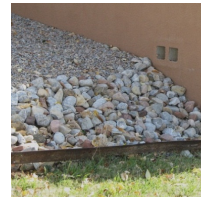
Image 4.16 Edging Installation Issues
