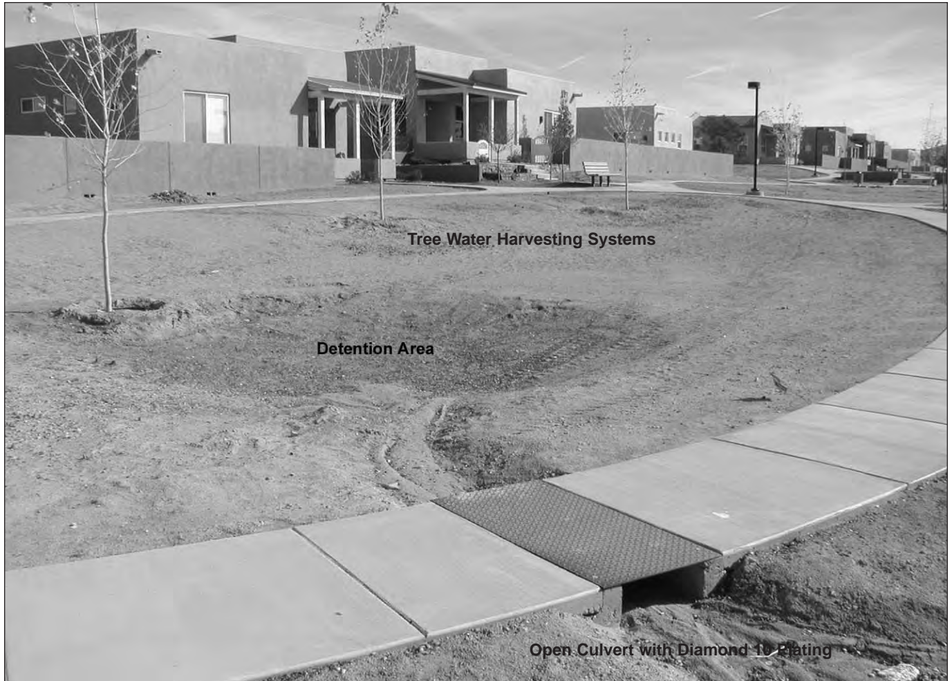
DRAINAGE WAY SIDEWALK CULVERT AT PARK OPEN SPACE (PRIOR TO GRASS INSTALLATION) WINDMILL RIDGE - UNIT 1 PARK
