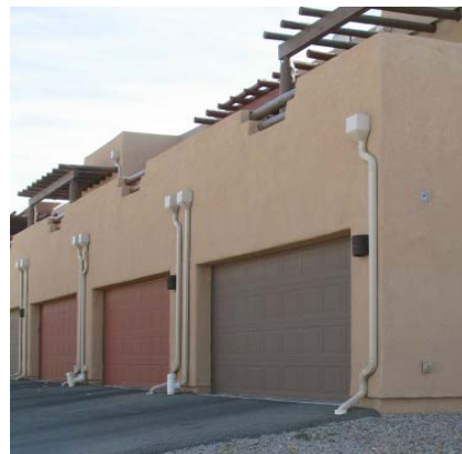
Image 4.10 Downspout to Underground Cistern
