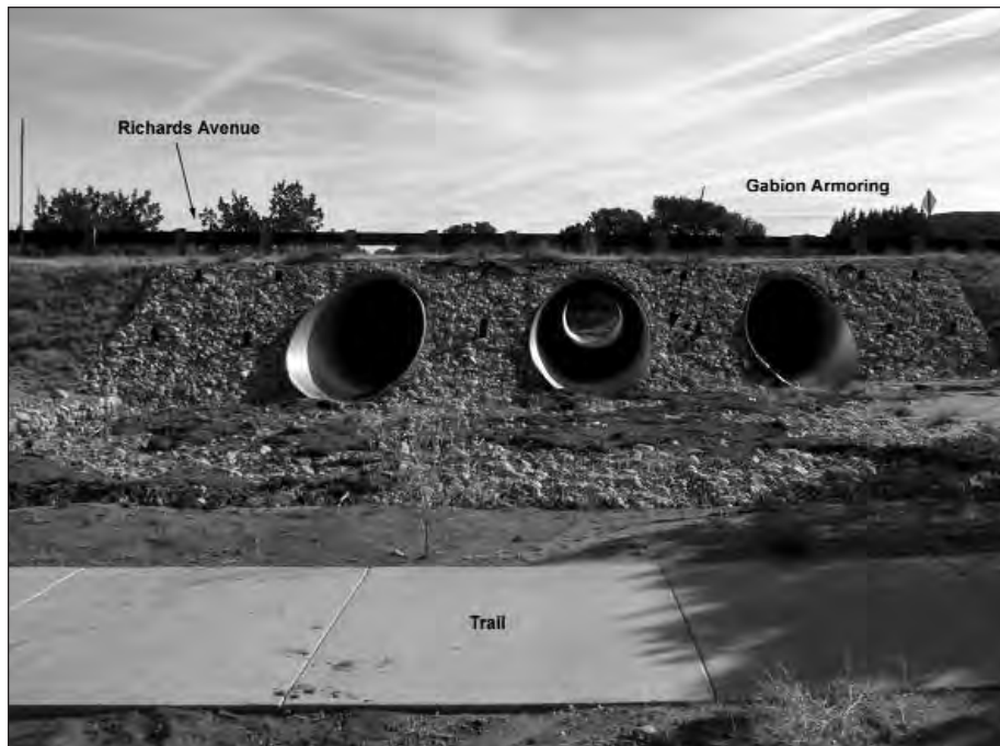
GABION AND ARMORING AT MAJOR ARROYO DRAINAGE WAY WINDMILL RIDGE - RICHARDS AVENUE
