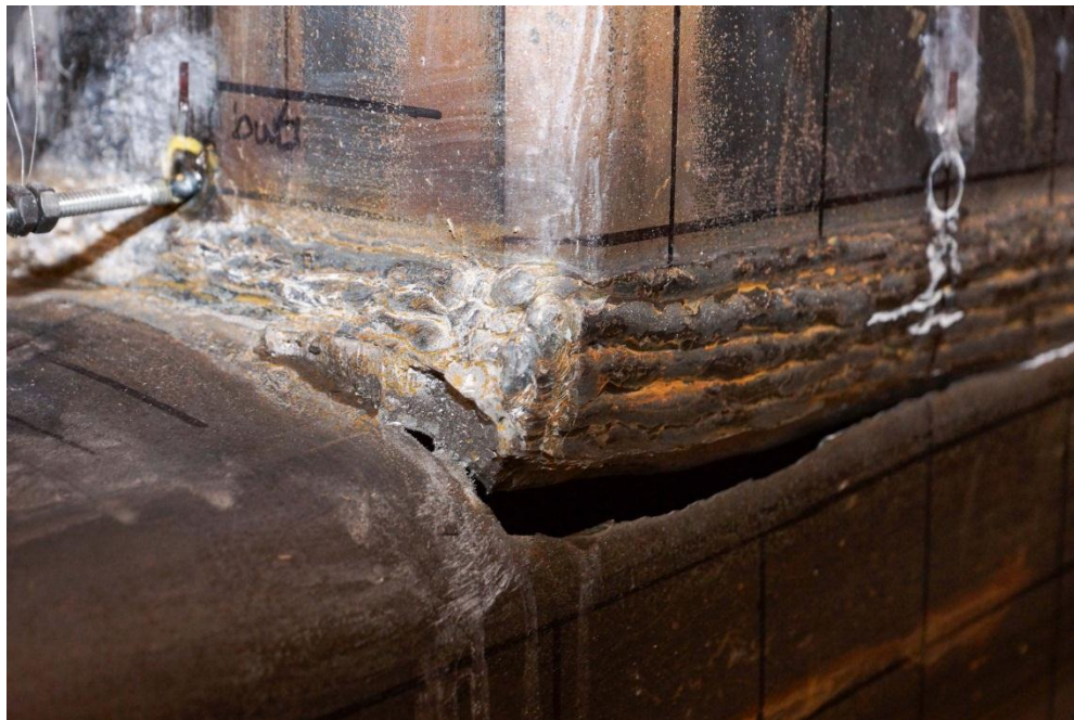
Figure 7.18 Close up of the fracture in the base metal of the column at the toe of the weld in the matched connection at the completion of the test
