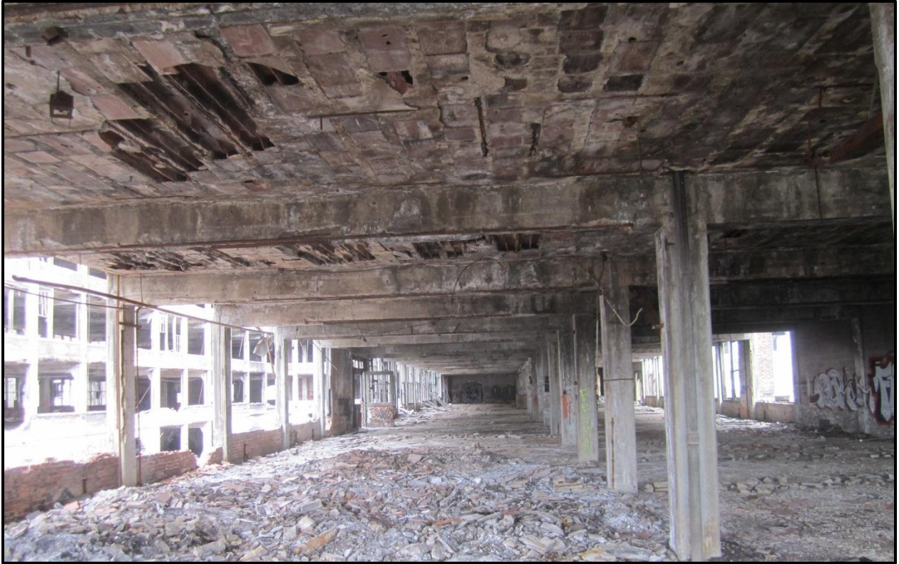
Figure 25. The Kahn System in situ.
