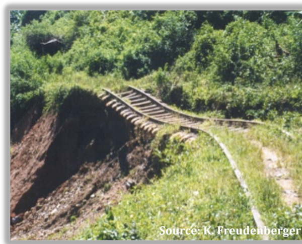
Figure 16 Washout along FCE in 2000
